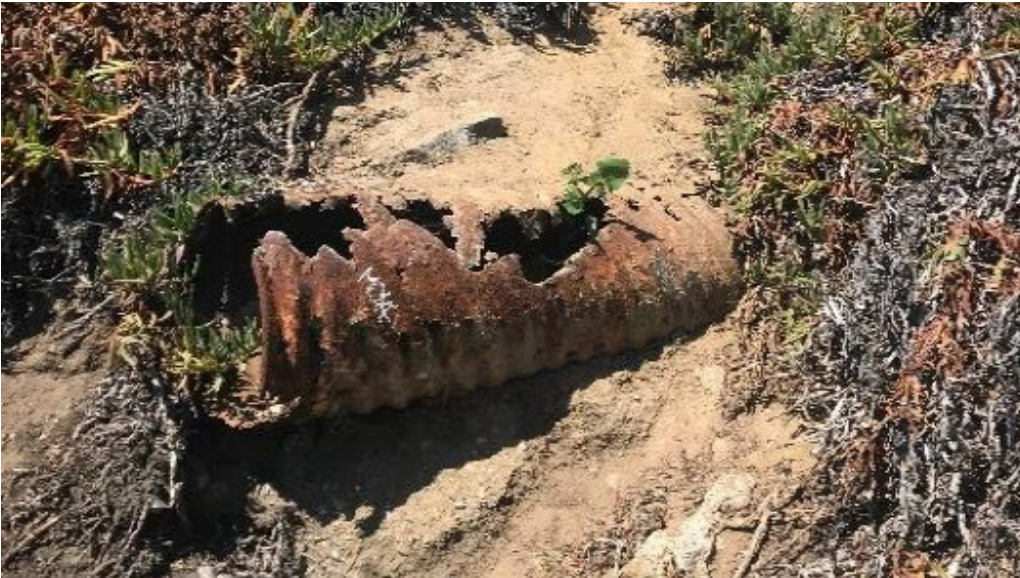
Example of stormwater outfall and proximity to erosion or seepage (source: City of Santa Cruz)
