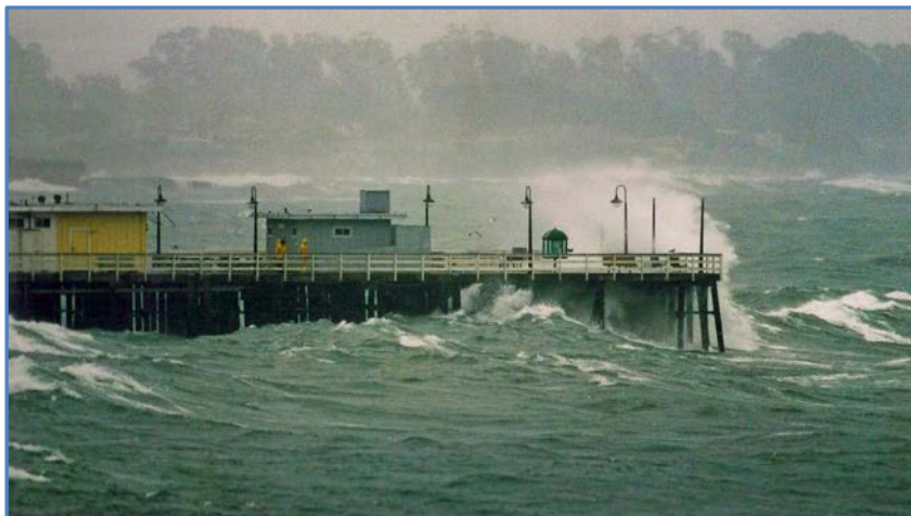
The Wharf's deck elevation of 23' (MLLW) puts it above all but the most extreme waves.
