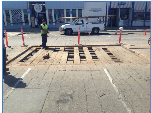
The roadway surface is subject to reflective cracking from below.
