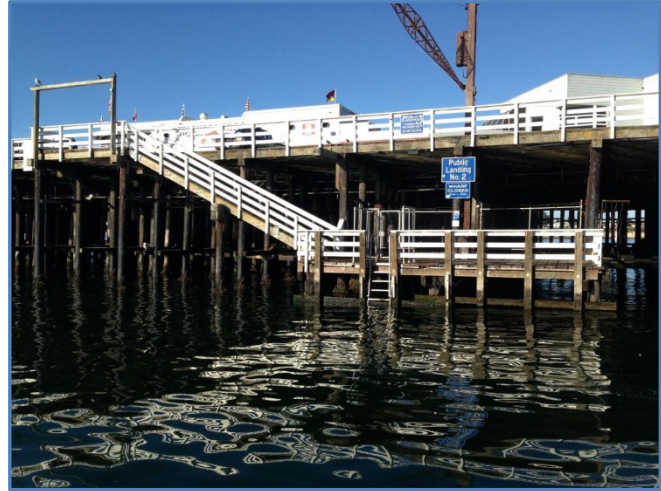
Public Landing No. 2 is available for public use for short term loading and offloading.
