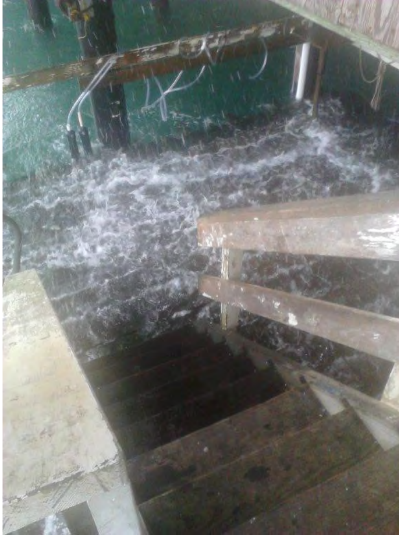
Photo 8-7: Wave Uplift at Existing Wharf Staff Landing
