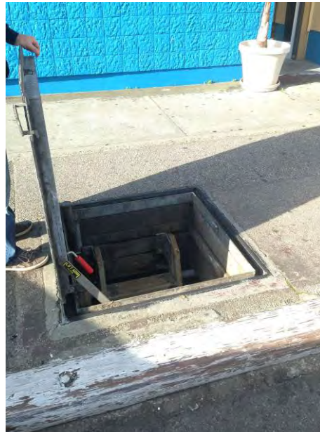
Photo 6-4: Fire Access Portal Bent 120
