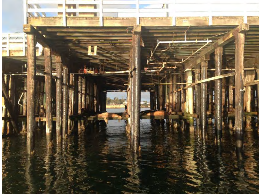
Photo 6-7: Sprinkler and BFP Bent 165
