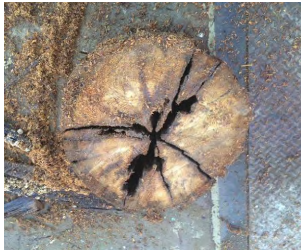
Photo 1-7: Pile with Teredo damage
