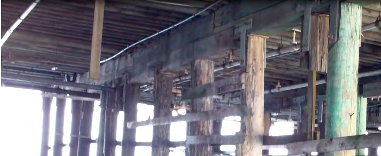
Photo 2-13: Long segment of double cap with multiple splices (Bent 165, looking east)
