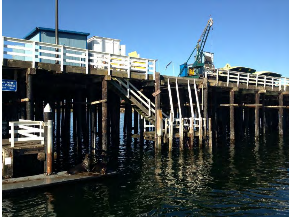
Photo 8-2: Boat Rental Hoist
