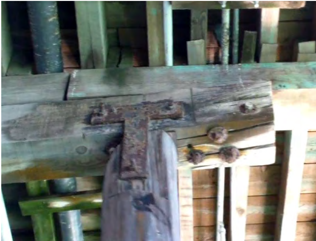
Photo 2-14: Cap Splitting at End – Bent 62, Pile 3
