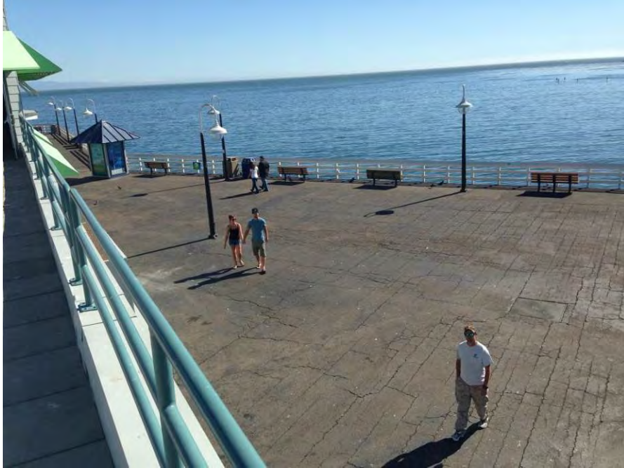
Photo 4-5: Pavement on South Commons
