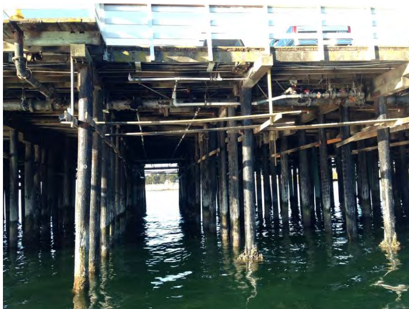
Photo 6-2: Fire Hydrant Bent 90
