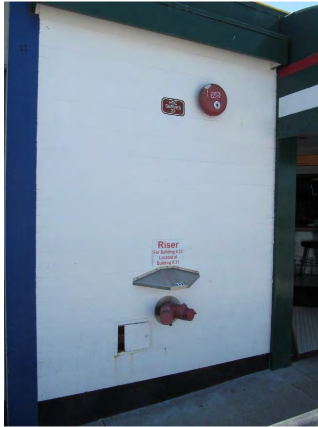
Photo 6-8: Typical Riser, Fire Department Connection, Bell, and Signage.
