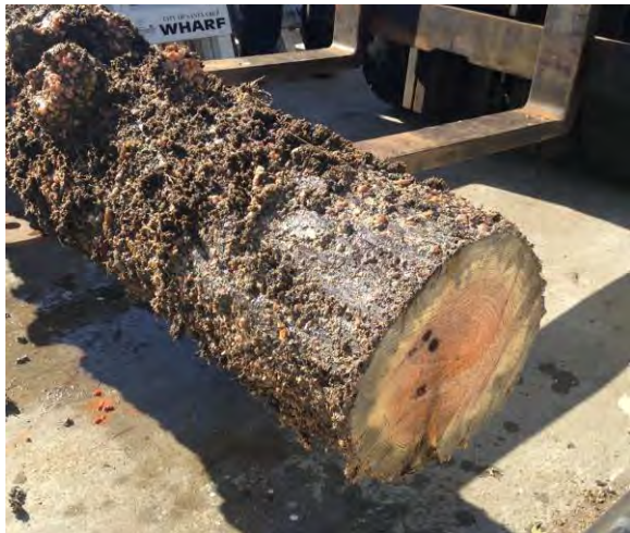
Photo 1-6: Pile with Teredo damage
