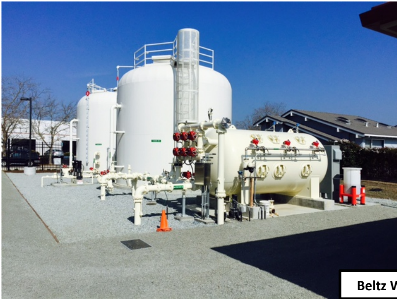
Bay Street Reservoir
