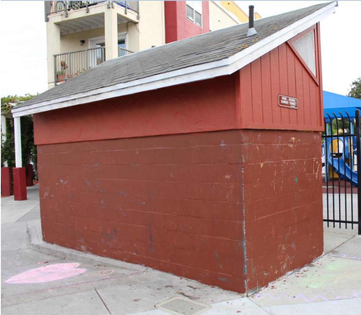
Beach Flats Park building after the vandalism of 9/11-14
