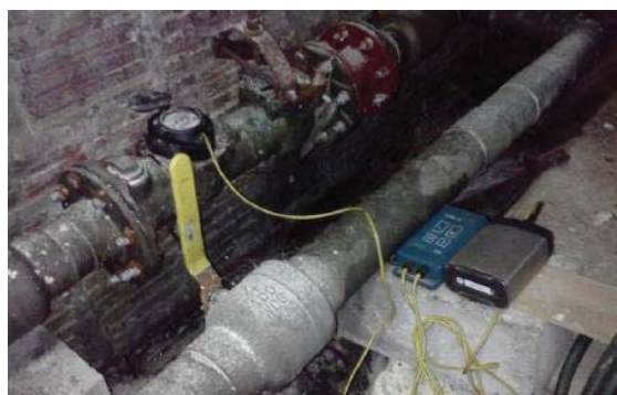
Figure 37: Meter-Master Installation and Data Logger – TRO Ave of the Arts
