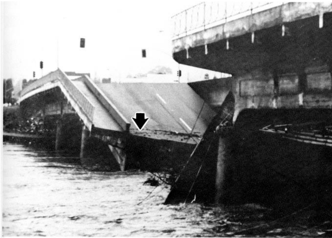
Figure 24. High flows in January 1982 in the San Lorenzo River scoured below the depth of the supporting piles leading to collapse of a portion of the Soquel Avenue Bridge. Arrow points to debris line from highest river flows.
