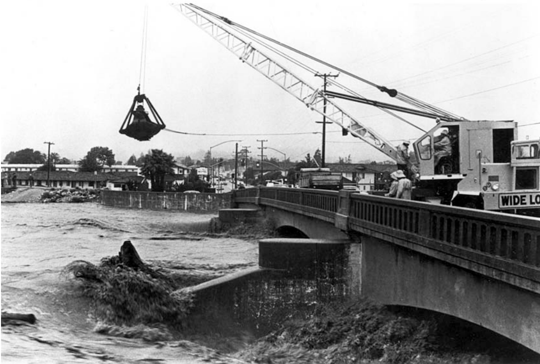
Figure 23. 1982 high water at former Riverside Avenue Bridge with crane removing logs and debris so as not to obstruct flow under the low arches of the old bridge.
