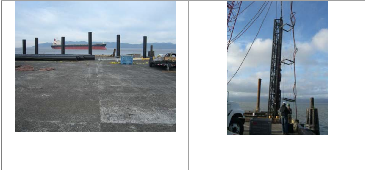
Figure 2a. Pile layout on Pier. Piles have been vibrated in and are ready to be driven with the impact hammer
