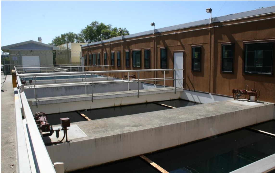
Figure 3: Existing Filters at the GHWTP
