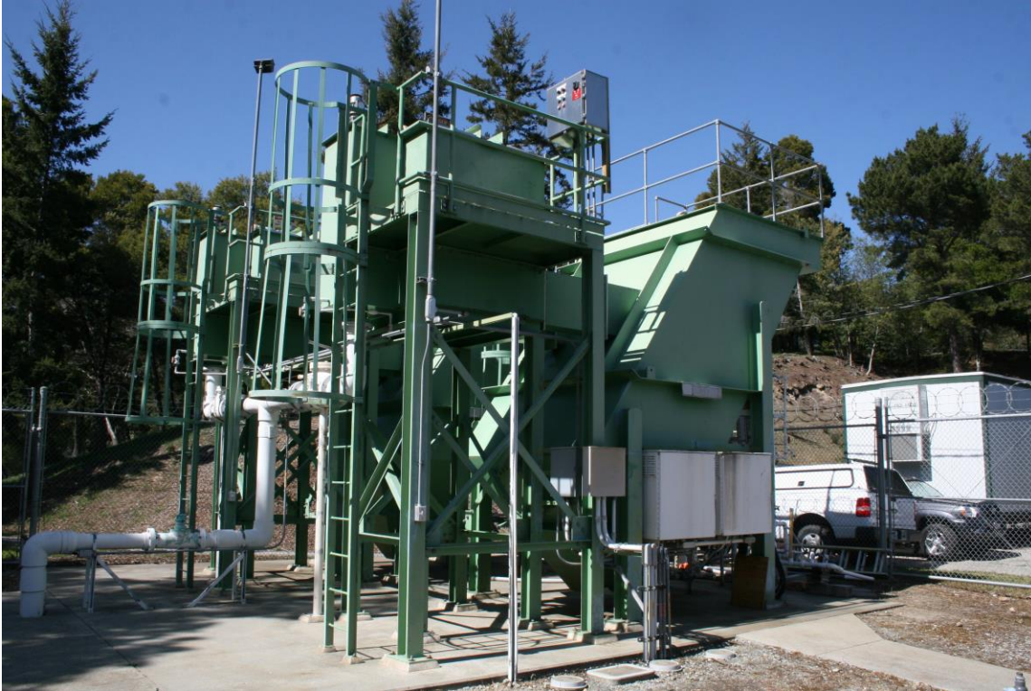
Figure 4: Existing Reclaimed Water Clarifier/Thickeners at the GHWTP
