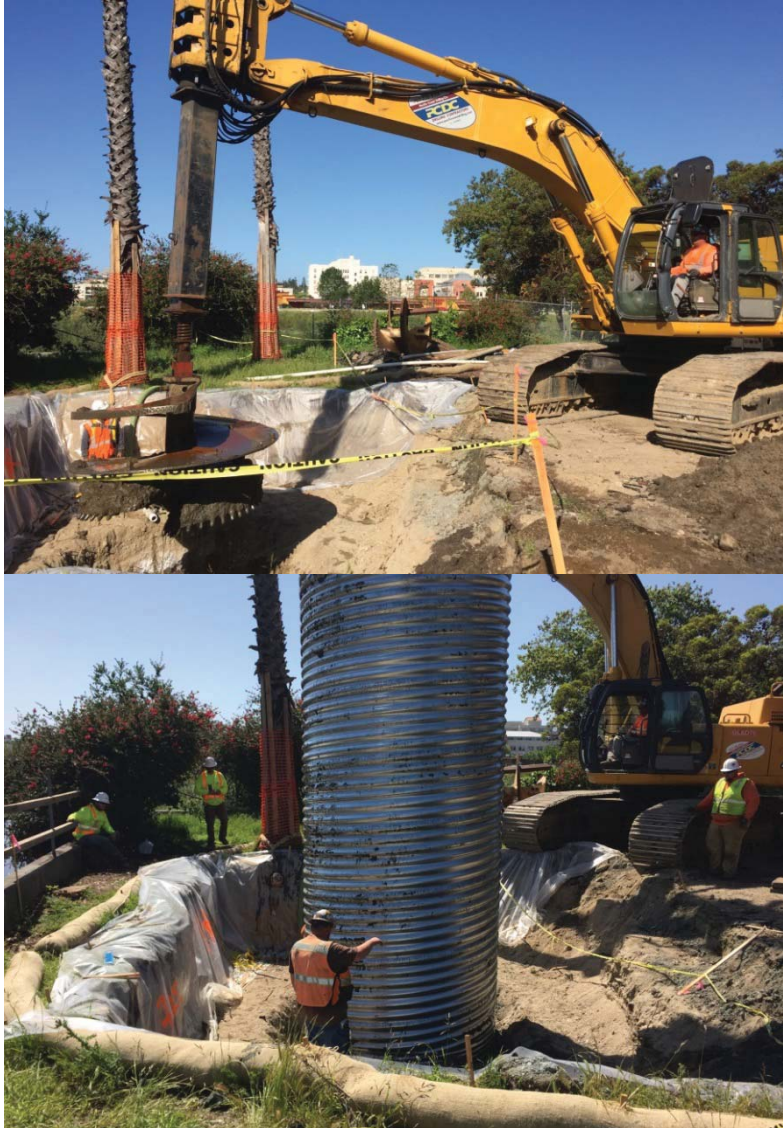
The Branciforte Bike/Pedestrian Bridge and Path under construction. This project will complete the “missing link” to the City’s 5.2 mile San Lorenzo River Levee.
