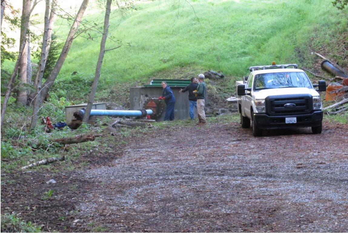
Outlet vault including deluge valve at Newell Creek Dam. (Continuous flow of water from reservoir is maintained for downstream environment.)
