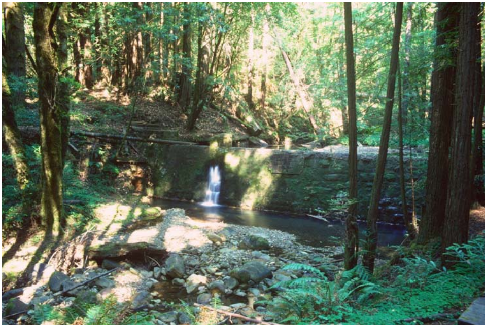
Creek Diversion Structure
