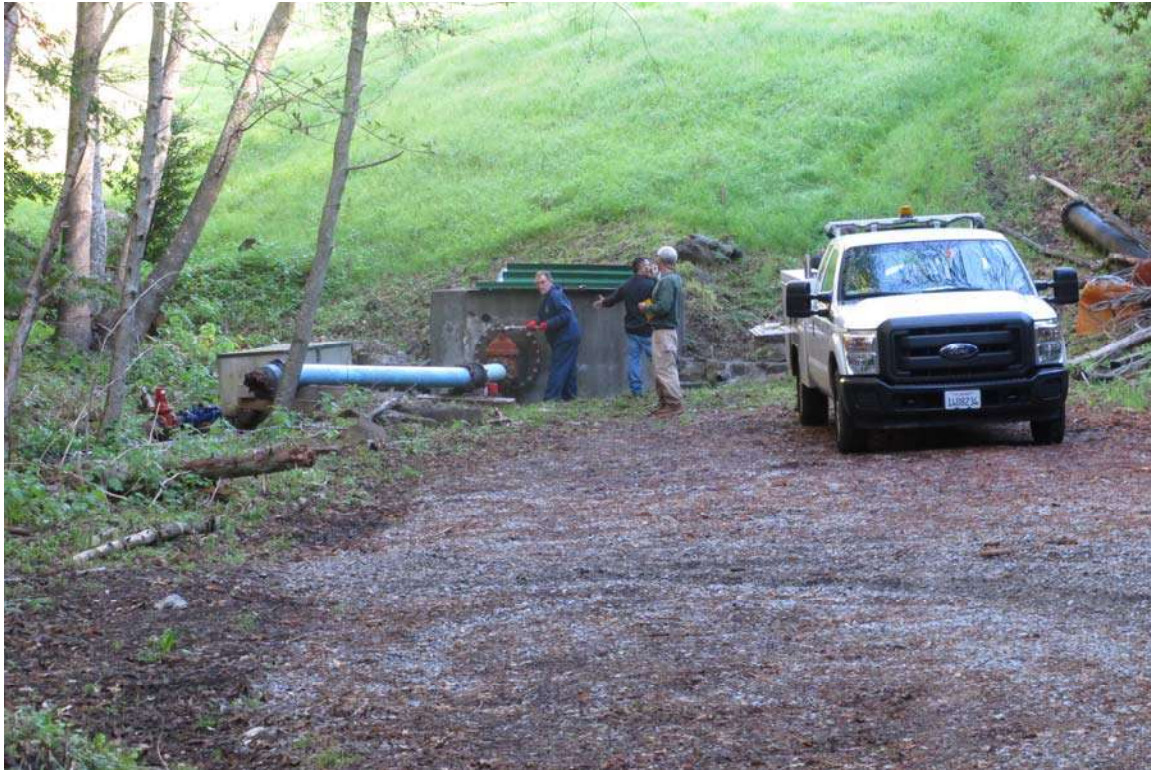
Outlet vault including deluge valve at Newell Creek Dam. (Continuous flow of water from reservoir is maintained for downstream environment.)
