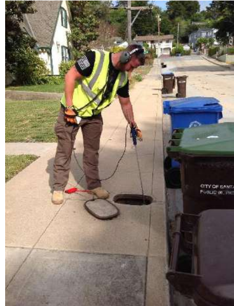
Figure 2: Sounding rod used in comprehensive acoustic leak detection
