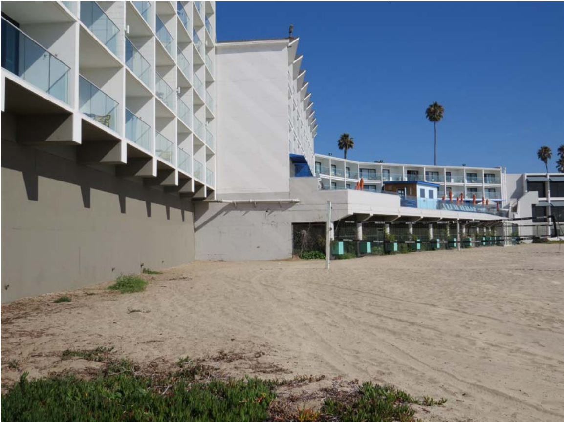
Figure 3. Protection of the bluff fronting the Dream Inn. The concrete wall on the left beneath the 10-story hotel portion spans 140 feet of hotel frontage. The restaurant on the far right is
