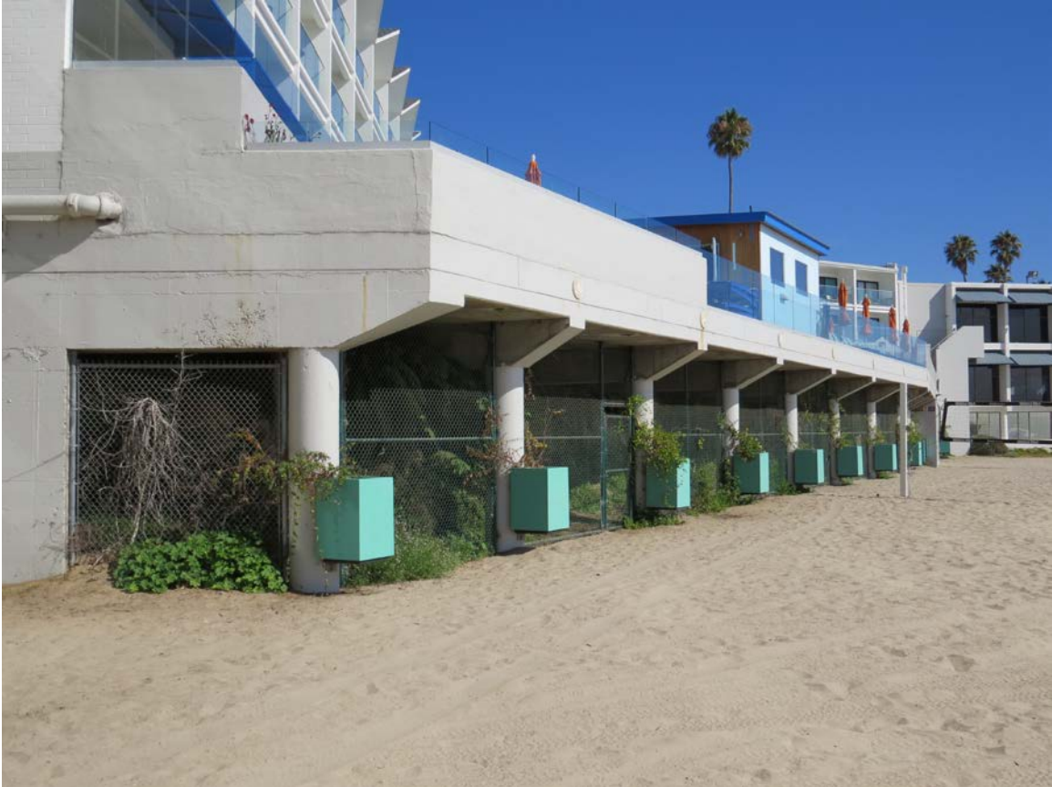
Figure 4. Area beneath the Dream Inn pool where Purisima Formation bedrock is exposed behind the row of concrete caissons and fencing.
