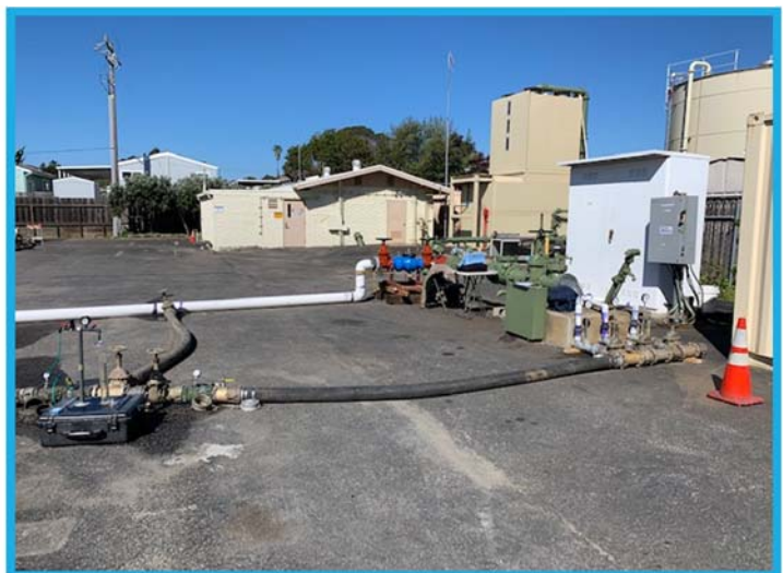
Figure 12 – ASR Pilot Testing at Beltz Well 8
