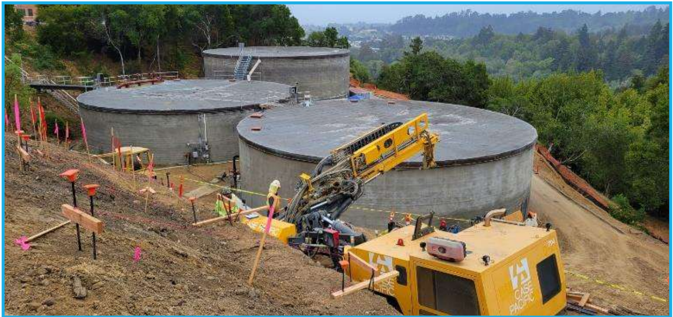
Photo 10: Graham Hill WTP Concrete Tanks Replacement – Soil nail installation and existing tanks
