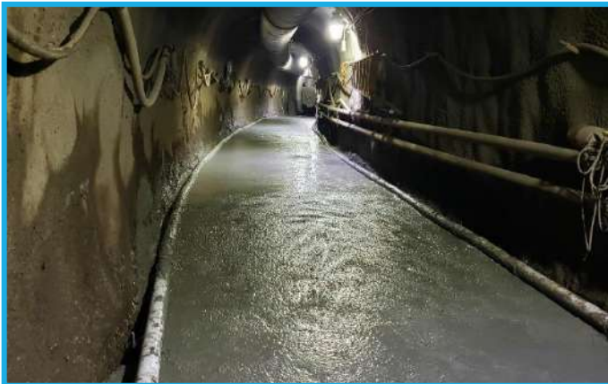
Photo 6: Newell Creek Dam Inlet/Outlet – Concrete pour for invert in tunnel for working slab
