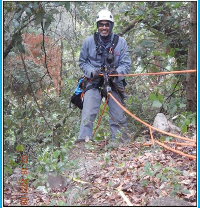
Photo 25: Ropes access used to inspect the pipes on a steep incline for U4 Tank pipes condition assessment
