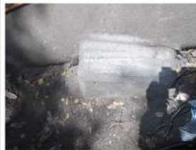
Figure 2-6. Station 0+63 Pipe Support Exposed West Side
