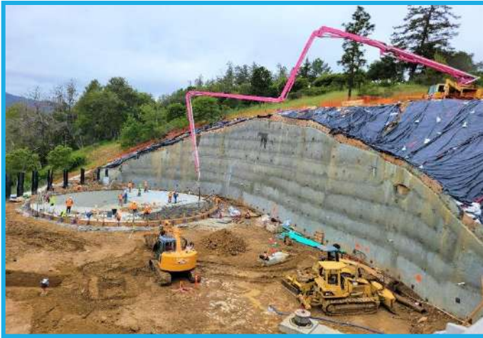
Photo 11: GHWTP Concrete Tanks Replacement Project - Residual Tank: Concrete Pouring from Pump Truck adjacent to Plant clarifiers. Slab and Slab Footing N-S quadrant looking SE
