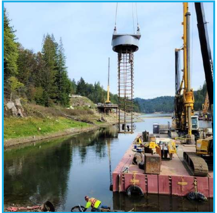
Photo 5: Using crane to lower rebar cage into Newell Creek Dam embankment CISS Piles
