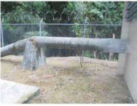
Figure 2-3. Exposed Pipe and Support Outside Pump Station No. 6
