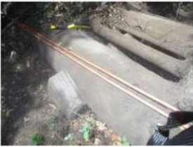
Figure 2-5. Station 0+63 Pipe Support Exposed Piping
