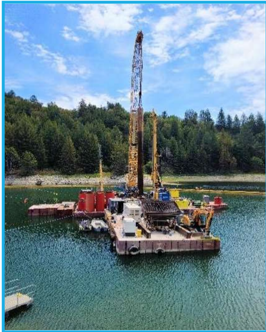
Photo 5: Lowering of steel casing for middle intake shaft at Newell Creek Dam
