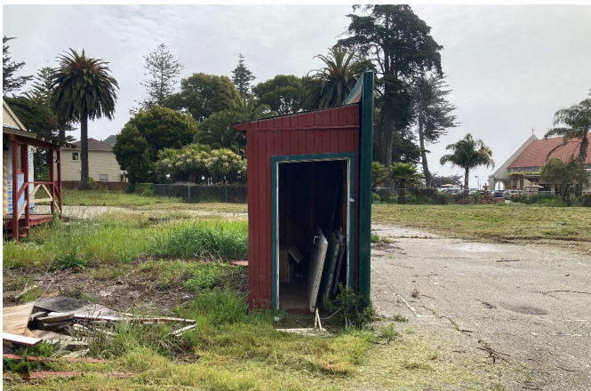
Figure 11: Wood-frame ancillary building, located to the south of the refectory building, looking east.
