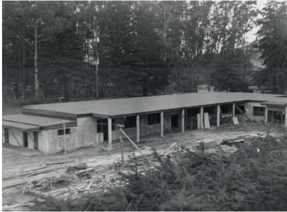
Figure 12: Original one-story chapel under construction in 1951. Source: Oblates of St. Joseph, online.
