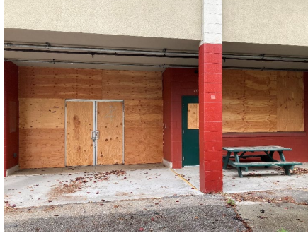
Figure 9: Recessed rear entry doors (set on same axis as the main entrance at the primary façade), looking west.
