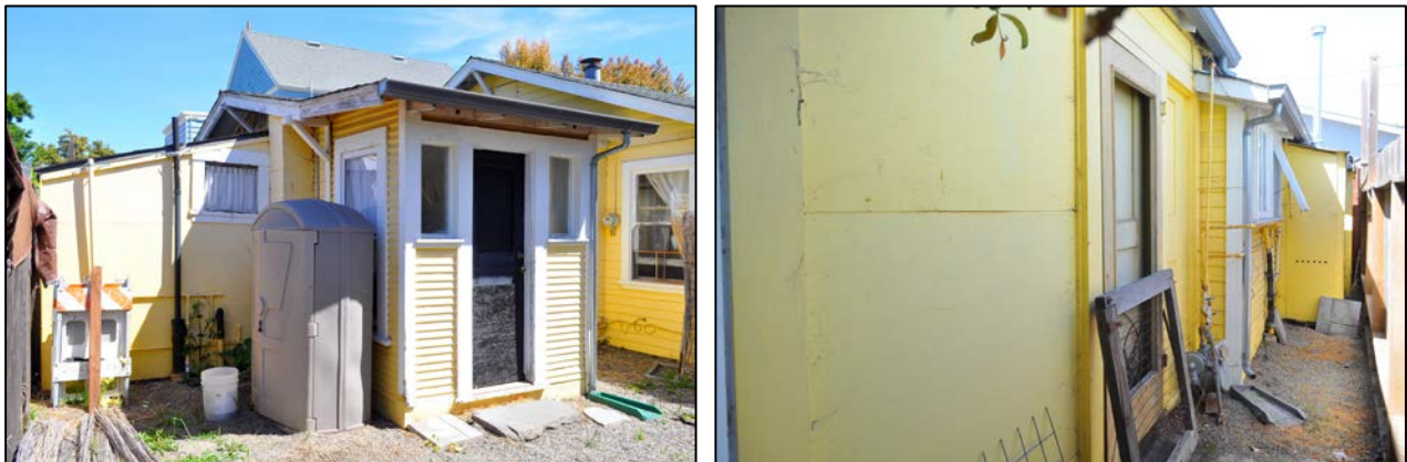
Figures 4 and 5. Left image shows the rear of the south elevation, with multiple additions. Right image shows the north elevation looking west, with windows covered by plywood and fenestration modifications.
