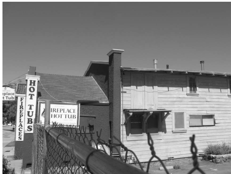
Photo 5: View of the southwest corner, showing transition between the store front and the remainder of the structure.
