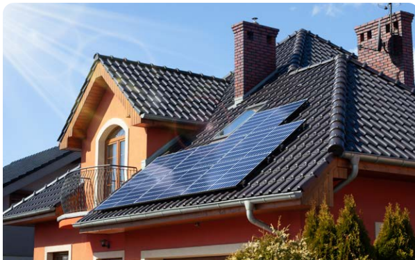
Residential Roof-mounted Solar Panels
