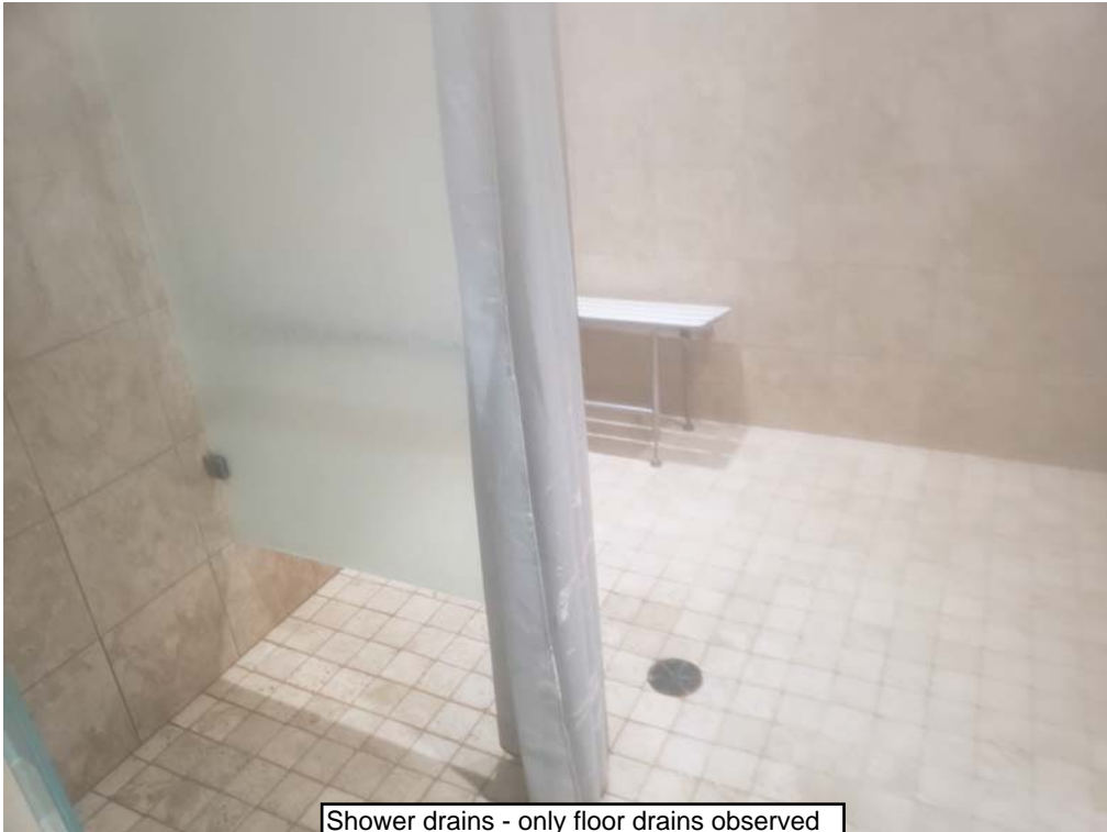
Shower drains - only floor drains observed
