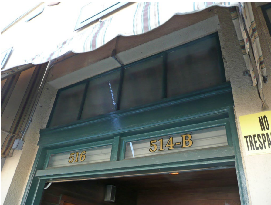
Detail of transom windows and clerestory windows above the recessed entrance in center bay on the west elevation.
