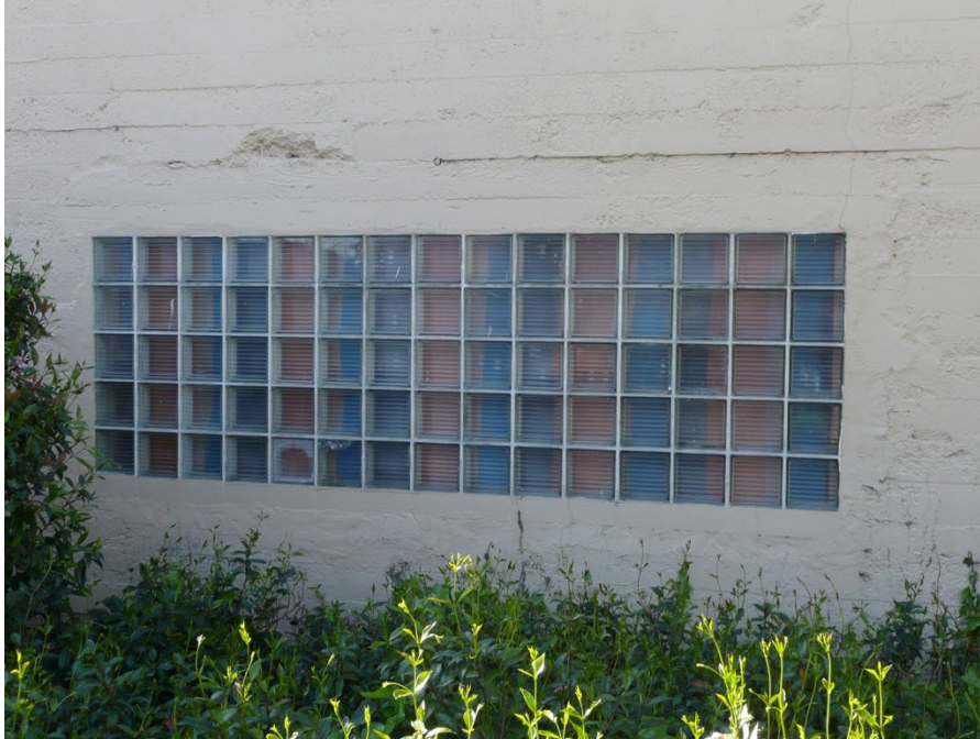
Detail of the cluster of glass blocks at the north elevation of the 1926 building, facing south.
