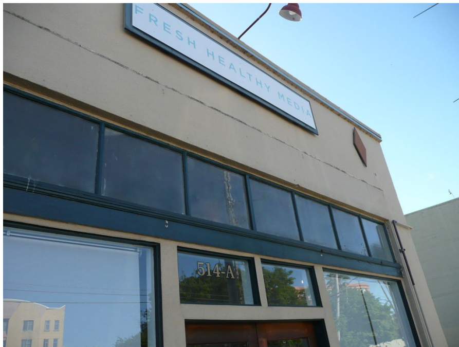
Detail of clerestory at the southernmost bay of the 1926 building, along the west elevation, facing southeast.
