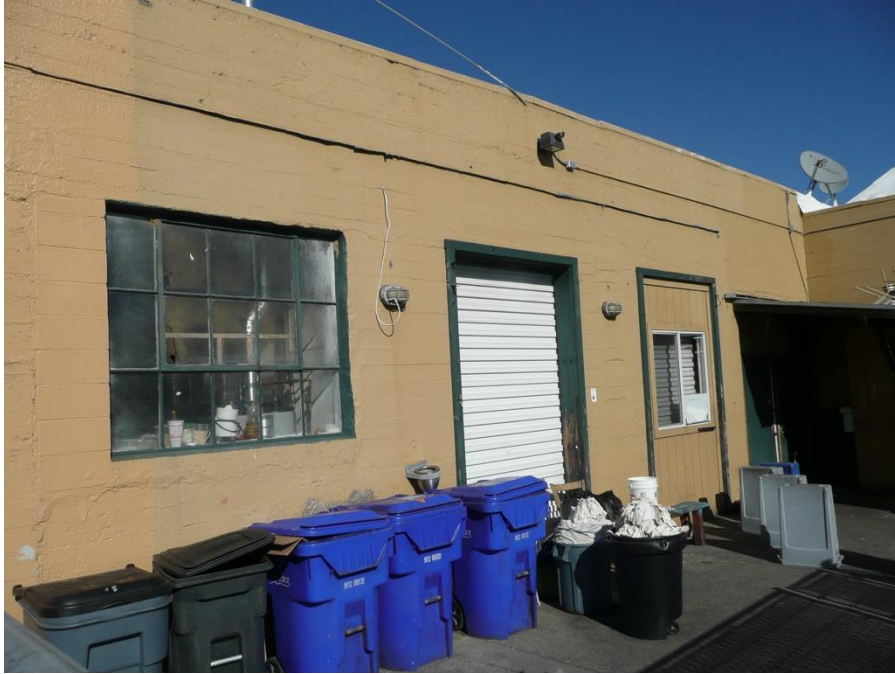
Figure 34: A portion of the east elevation of the main building form, showing one of the two multilight windows at left, the roll-up garage door at center, the infilled garage door with window at right, facing northwest.
