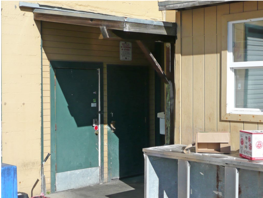
Detail of rear entry doors at the east elevation of the main building form, facing northwest. The contemporary shed-roof addition at the south elevation of the rear wing is also visible at right.
