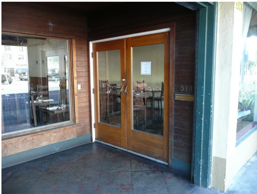
Figure 19: Detail of recessed opening within the center bay, showing the plate-glass window and north-facing double doors facing southeast.
