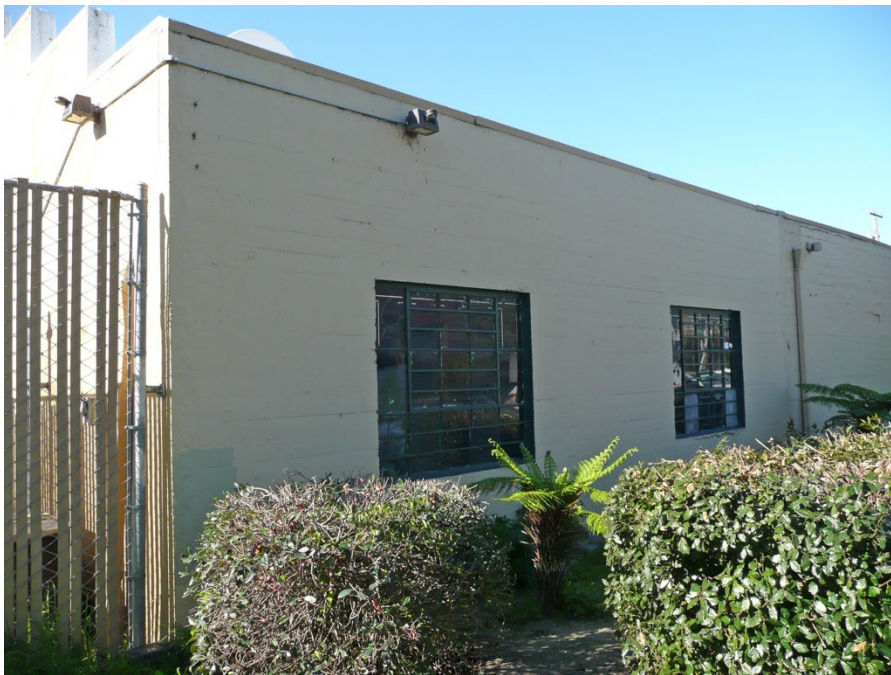
Detail of the two metal multi-light windows near the eastern end of the north elevation of the 1926 building, facing southwest.
