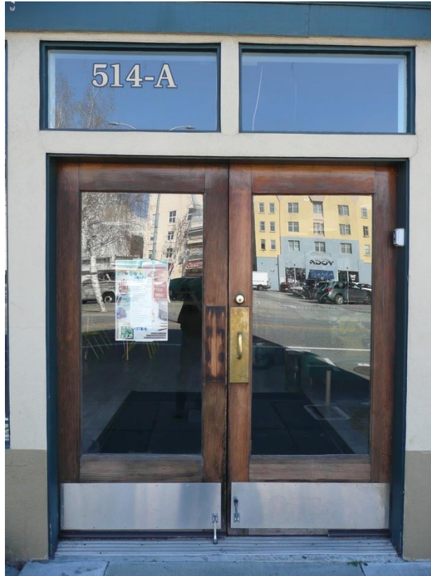
Figure 14: Detail of the contemporary doors and transom windows at the southernmost bay of the 1926 building.
