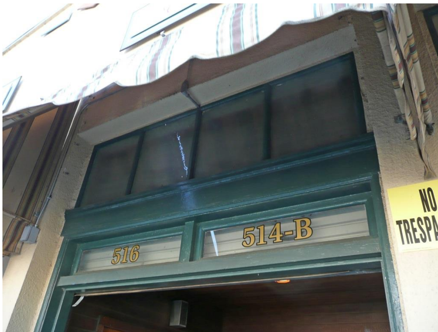
Figure 17: Detail of transom windows and clerestory windows above the recessed entrance in center bay on the west elevation.
