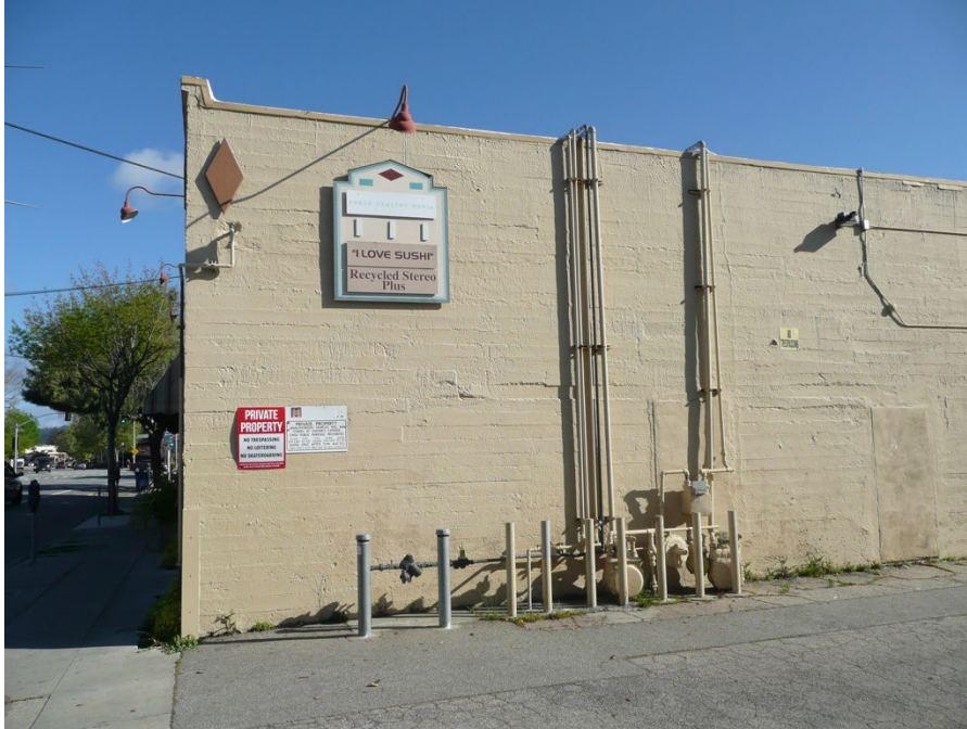
Western corner of the south elevation of the main building form, facing north.
