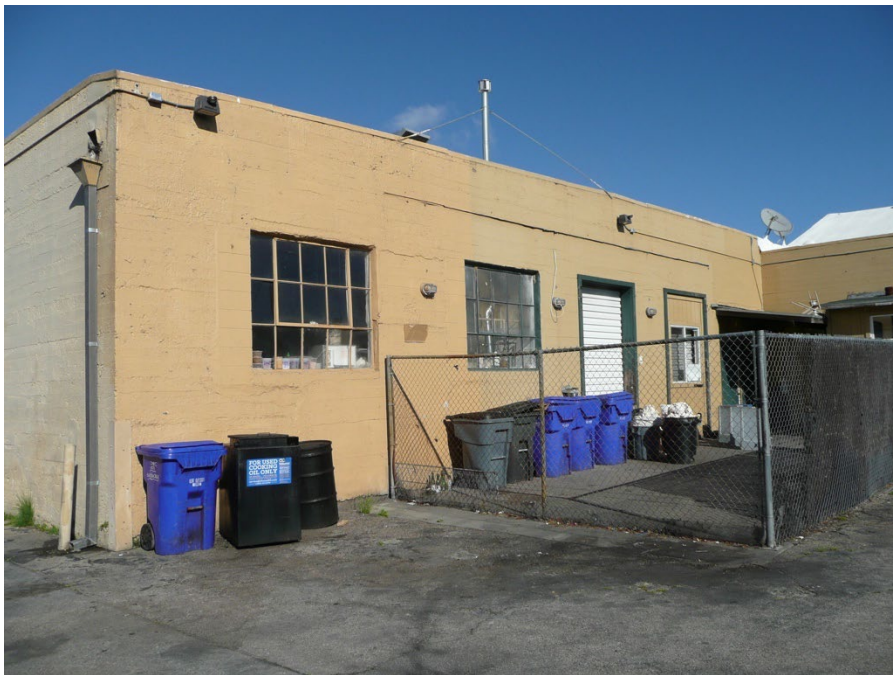
East elevation of the main building form, with the south elevation of the rear wing visible at far right, facing northwest.
