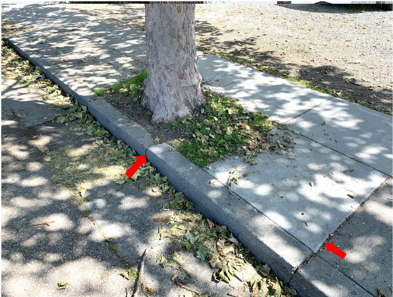
Image #3 - Tree T3, London plane. Note lighter colored concrete is more recent. Also lifting of sidewalk and curb cracking (arrows).
