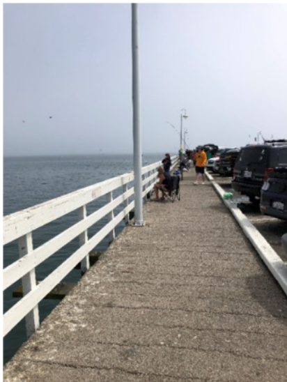
“Tailgate” Fishing on East Side of Wharf that Encroaches into Pedestrian Walkway
