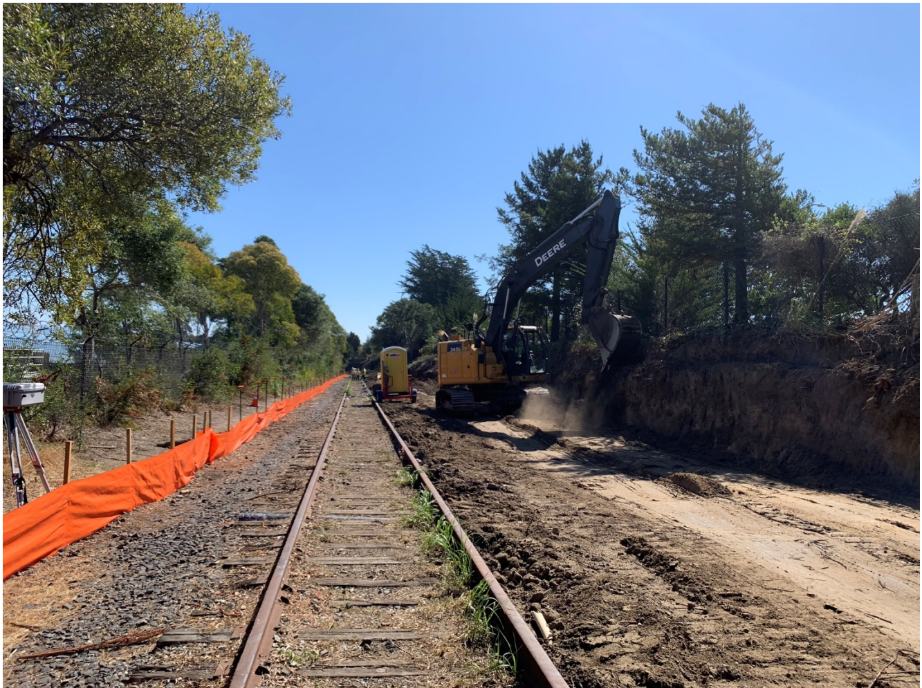
Figure 1 Construction of Segment 7 of the Monterey Bay Sanctuary Scenic Trail (Rail Trail).
