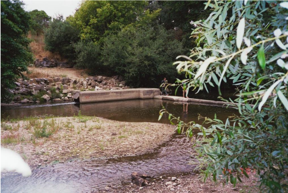
Photo: Tait Street Diversion from left bank downstream looking across the channel
