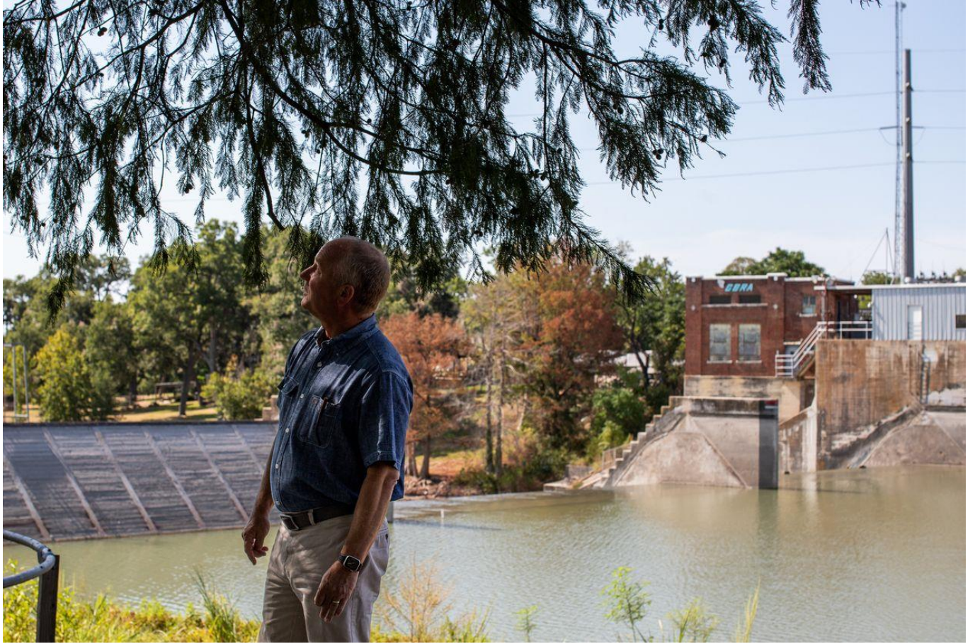
Paul Mueller watching a construction crew make repairs to the spill gates on the McQueeney dam.
