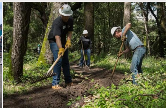
Trail crew members hard at work constructing the Emma McCrary trail in Pogonip Open Space. This was the city's first collaboration with the group in 2012.
