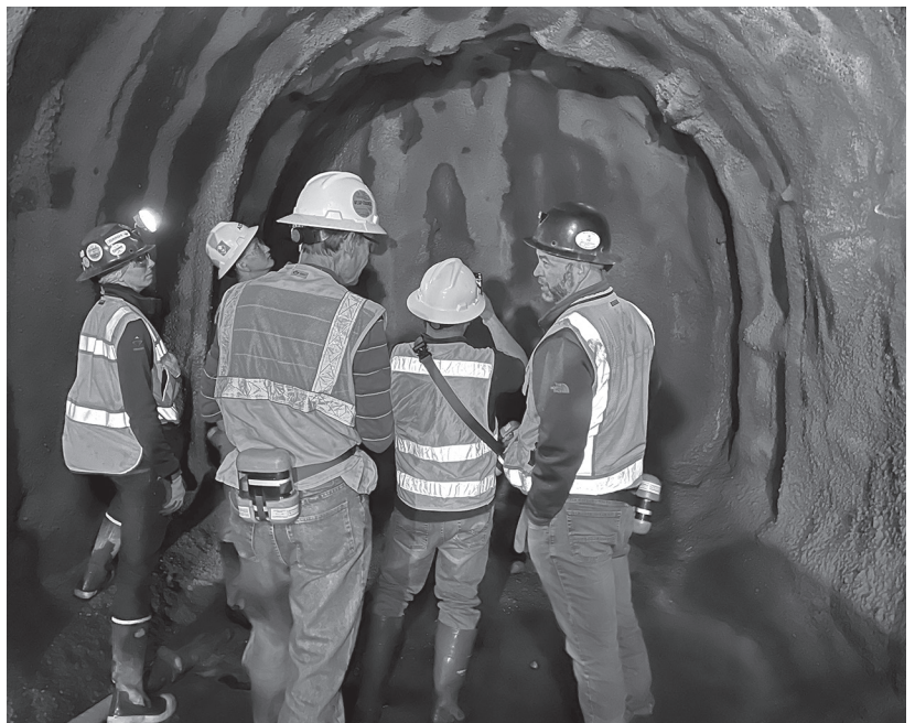
A team of staff and contractors tunneled around the dam and under the reservoir to connect to brand-new intake structures to replace the old infrastructure.
