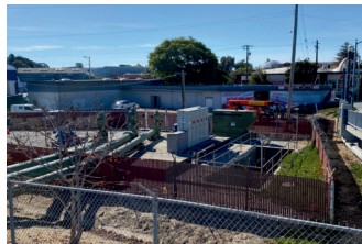
Stormwater Pump Station No. 1 and Soquel Pump Station
